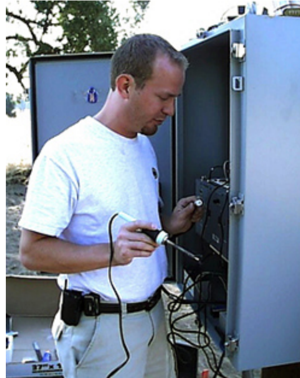
Information Station Specialists' Field Tech Tom Coviak installs a Travelers Information Station. Photo courtesy Information Station Specialists
