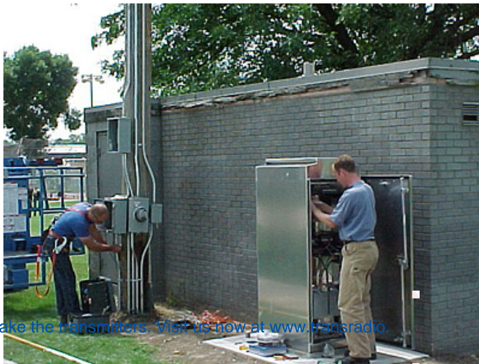
Mike Kattich from Century Electric and Tom Coviak from Information Station Specialists install electronics and route services for a TIS station in Aurora, Ill. Photo courtesy Information Station Specialists
